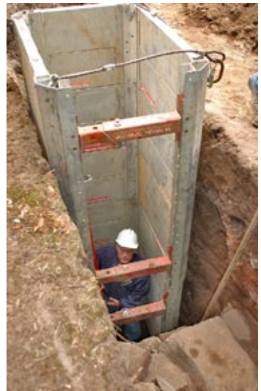
Tom Fowler of Miller Engineering inspects the east side of the foundation from the safety of a shoring box.
